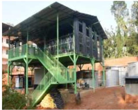
1 MLD STP at Kozhikode medical College
