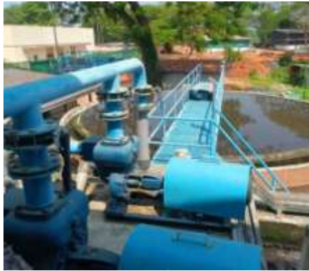
500 KLD STP at Kozhikode medical College
