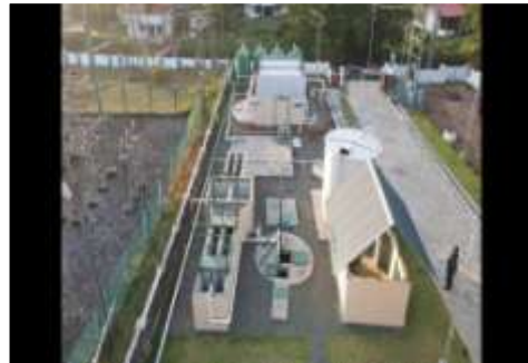
1 MLD CSTP at Padanappalam, Kannur
